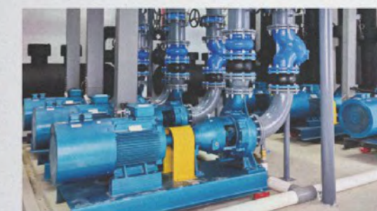
循环水泵 Circulating Water Pump
